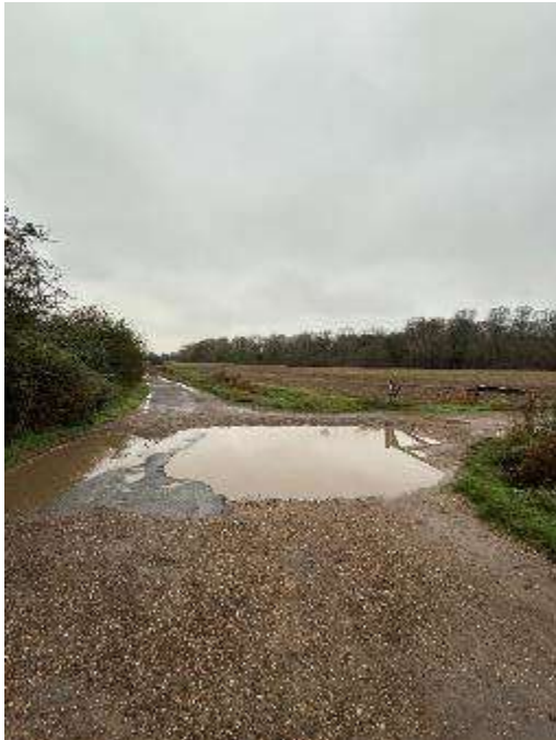
Standing water and pooling associated with inadequate drainage and maintenance, increasing safety risk and reducing usable carriageway width.
