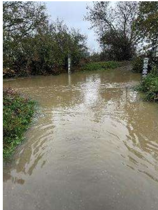
Ford crossing at Hail Weston, prone to regular flooding and temporary closure, presenting a foreseeable obstruction to vehicle movement and emergency access.
