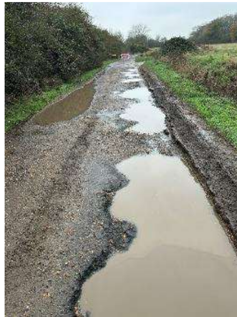
Road surface condition showing degradation and limited structural capacity, unsuitable for sustained HGV or construction traffic.
